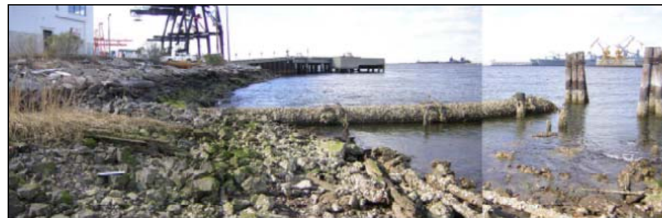
PHOTO 7: 30-inch diameter water pipeline landfall on Portsmouth shore. View is looking downstream (northwest).
